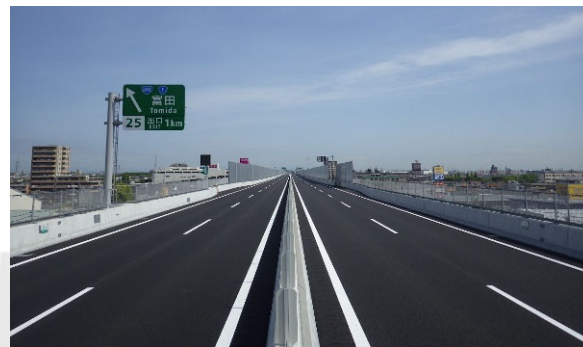
Pavement construction work between Nagoya-nishi Junction and Asuka Junction on Mei-Nikan Expressway
