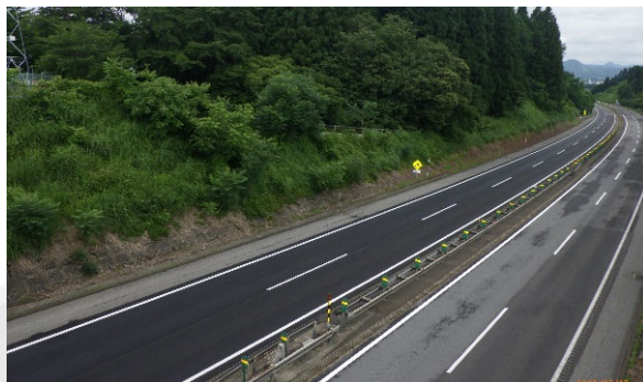
Pavement repair work within the jurisdiction of Towada Management Office of Tohoku Expressway
