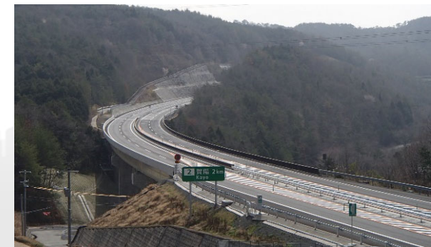
Pavement construction work between Okayama Junction and Ukan Interchange on Okayama Expressway
