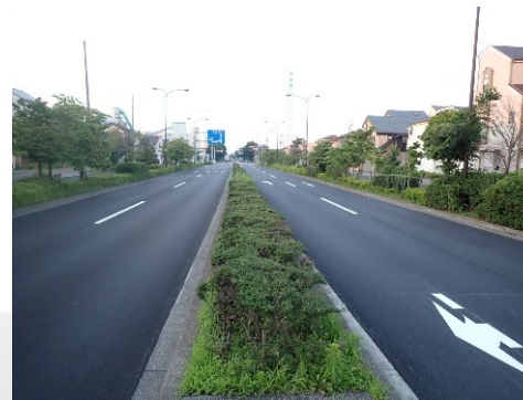
Surface repair work (FY2021, Kita-Tama South-6, two-layer low-noise pavement) and road sign installation work (FY2021, Kita-Tama South-1)
