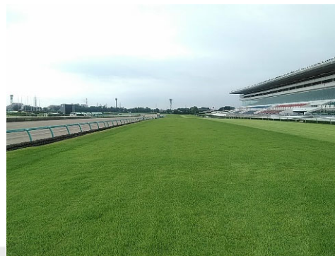
Nakayama Racecourse roadbed reconstruction work on the front turf road (4th corner side) and turf replacement work on the turf road
